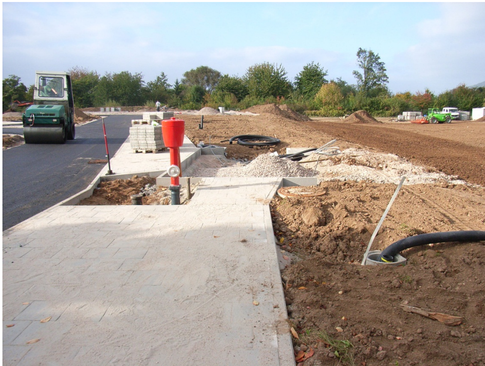
access to helipad with hydrant
